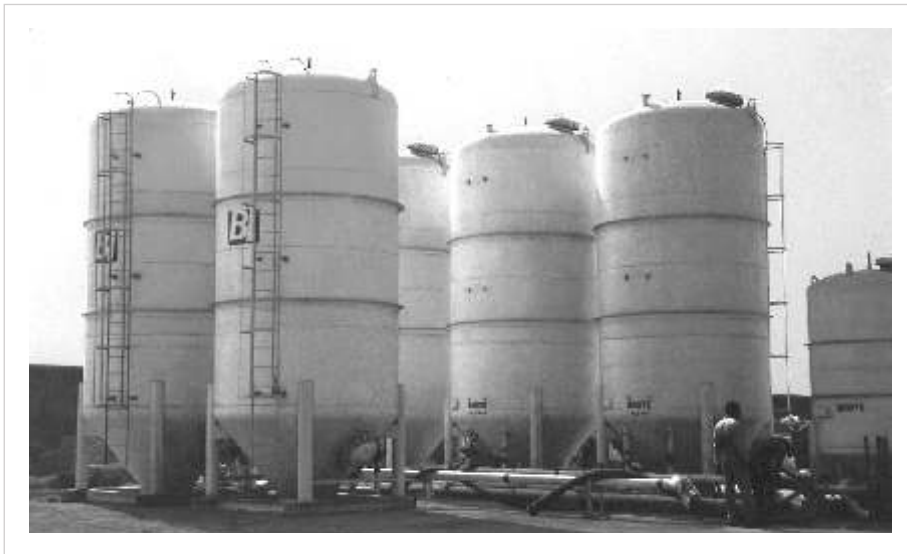
INSTALLED BULK PLANT AT VIZAG CLIENT : BJ SERVICES MIDDLE EAST INDIA LTD.
